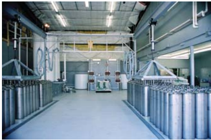
Inside the Blair Water Conditioning plant in Safety Harbor, Florida
